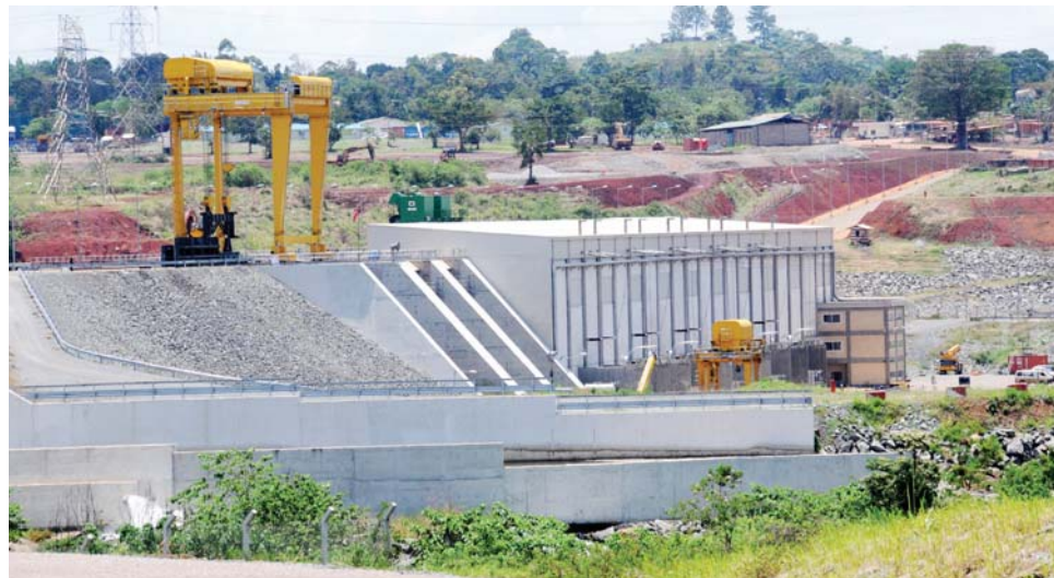
Bujagali hydro-power plant. The new hydro-power plants will add 33MW on the national grid
