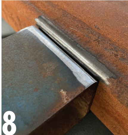
8 The same applies with two sections of RHS placed side-by-side where the corner radius forms a sufficient preparation for welding, provided it has been cleaned up. This is known as a V-groove flare joint.
