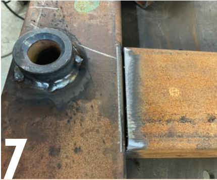
7 Sometimes joint design requires little additional edge preparation other than grinding off mill scale and rust. The thick-wall RHS section above has a natural radius providing sufficient preparation when the square edge of another section is butted up against it. This is known as a bevel flare groove. For a thicker square edge, a V-prep may be necessary to achieve full penetration (flare-V preparation).
