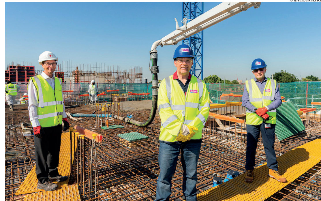
Cllr Rodwell (centre) during the early stages of the Sebastian Court housing development in Barking & Dagenham (along with William Jerram of Jerram Falkus and Iain Ferguson of Be First)
