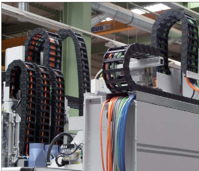
Permanently reliable data transmissions, e.g. with chainflex® cables harnessed to DriveCliqu standard.
